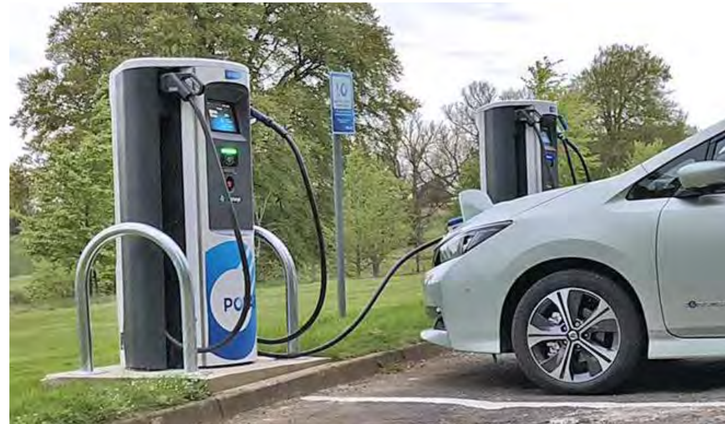
Electric charging point for vehicles.
