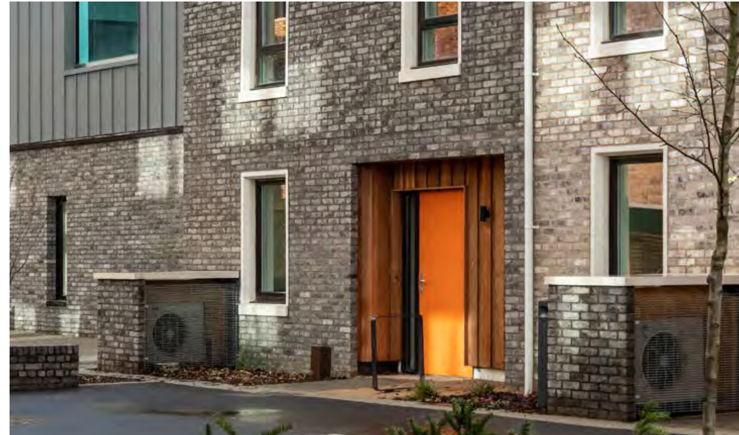
Air Source Heat Pumps
