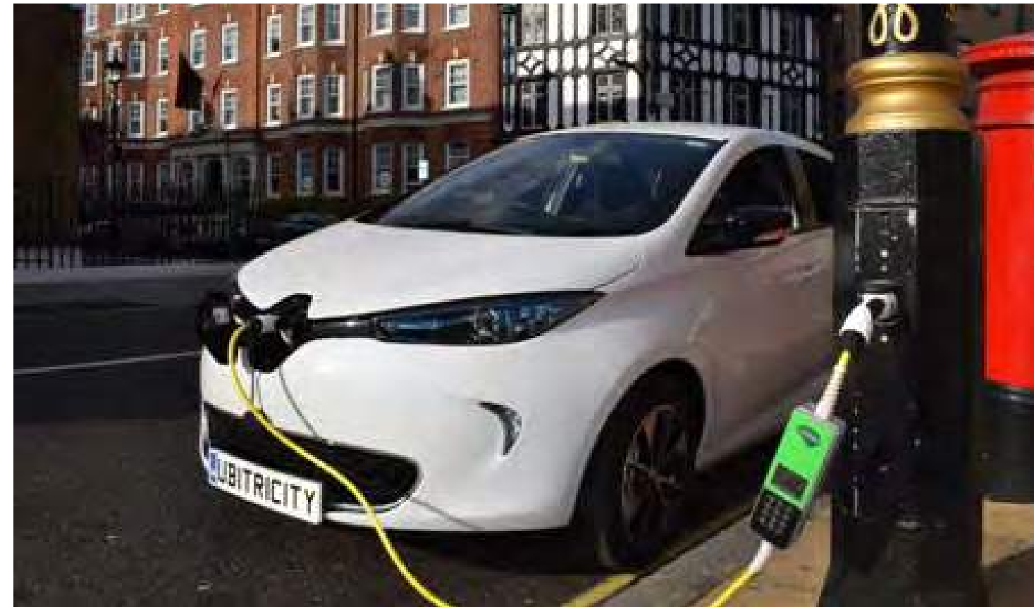
Electric charging point integrated with street furniture.
