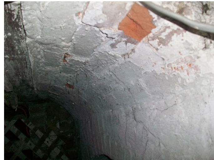
Left: Ventilated storage area - bridging and joists visible with repairs
