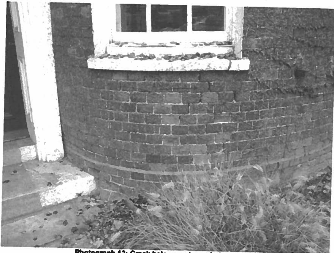
Photograph 12: Crack below western window of bay
