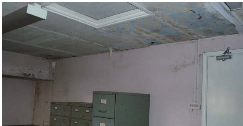
Talking newspaper (West) – serious damp to ceiling
