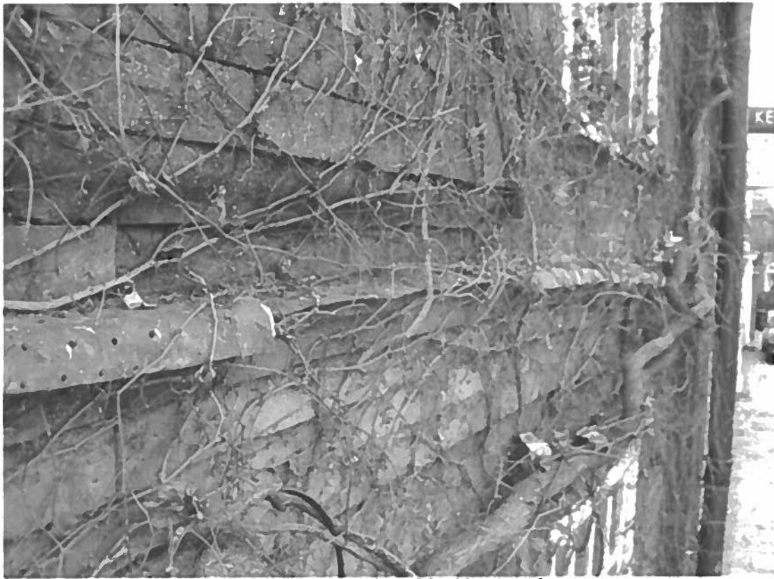
Photograph 5: Missing section of flashing to string course
