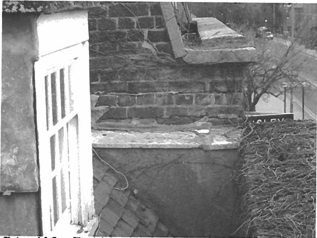
Photograph 9: Foam filler at abutment with adjoining building to east and missing flashing(?)
