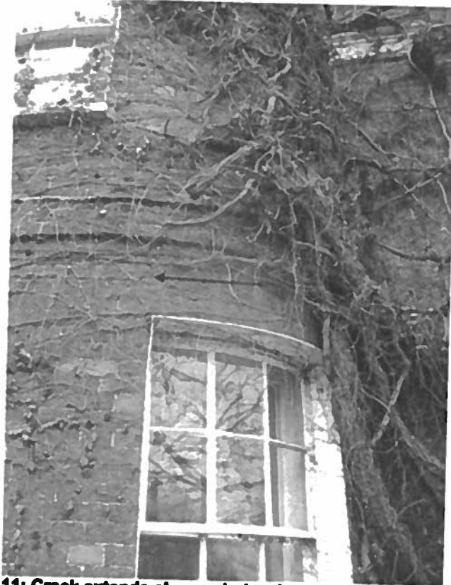
Photograph 11: Crack extends above window but partial concealed by creeper
