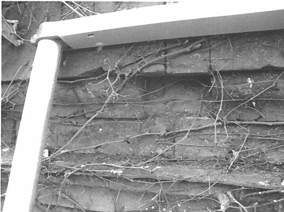
Photograph 8: Locally decayed bricks,
