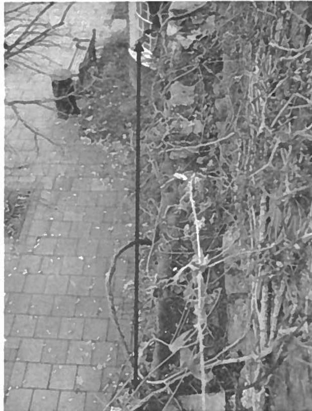
Photograph 6: Missing length of cornice flashing
