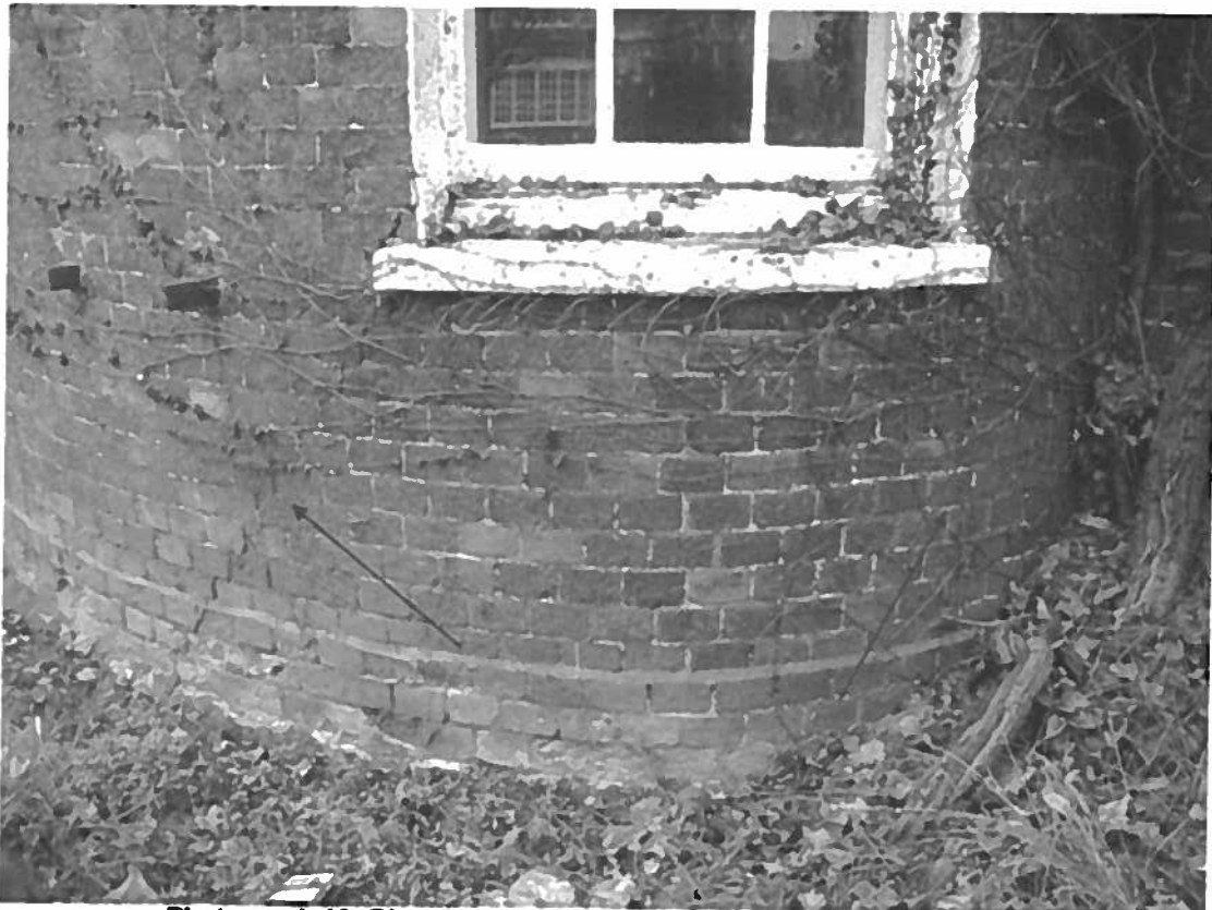
Photograph 10: Diagonal raking cracks below eastern window of bay
