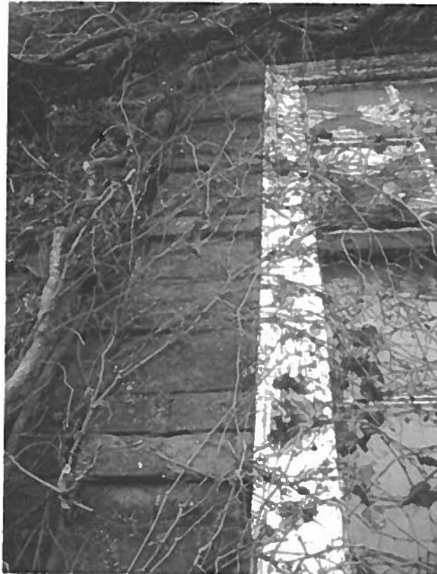
Photograph 4: Set forward brickwork adjacent to window reveal found to be loose
