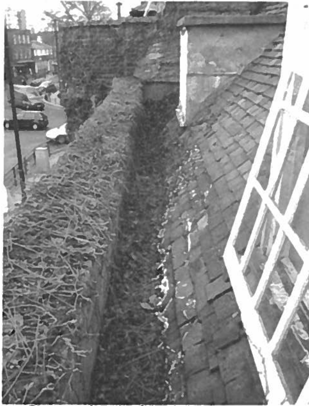
Photograph 7: Leaf debris in parapet gutter
