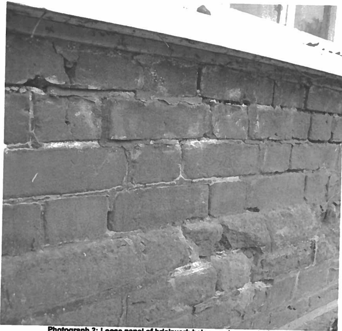
Photograph 2: Loose panel of brickwork below easternmost window
